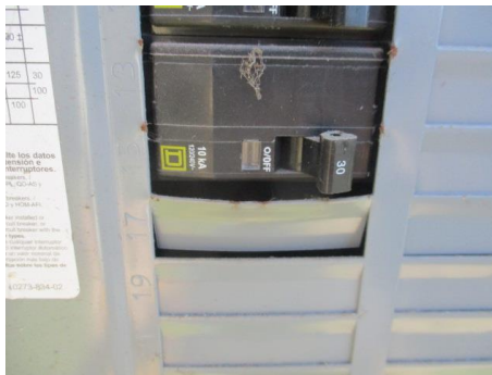
Damaged knock out in the main panel.
