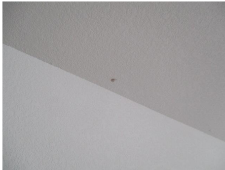
Nails backing out of the ceiling in the bedroom. Damaged and stained carpet.
